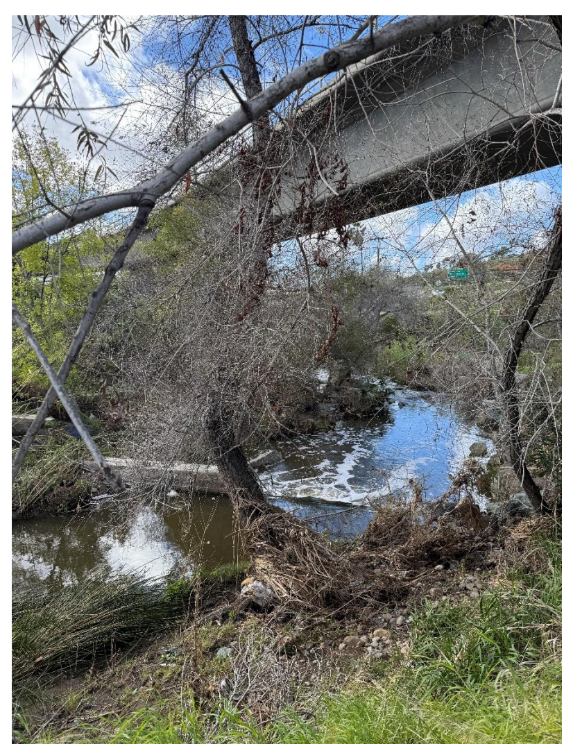
Image 2: Scour pool seen downstream of survey area.
