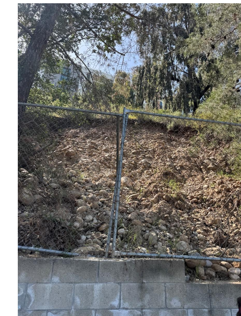
Image 6: Construction fence on east side of campus housing, holding back rocks from mass wasting slide event.
